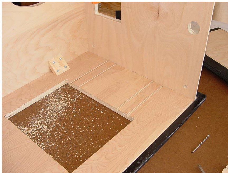
Installing the left side of the cabinet. Notice the corner gusset for added strength.
